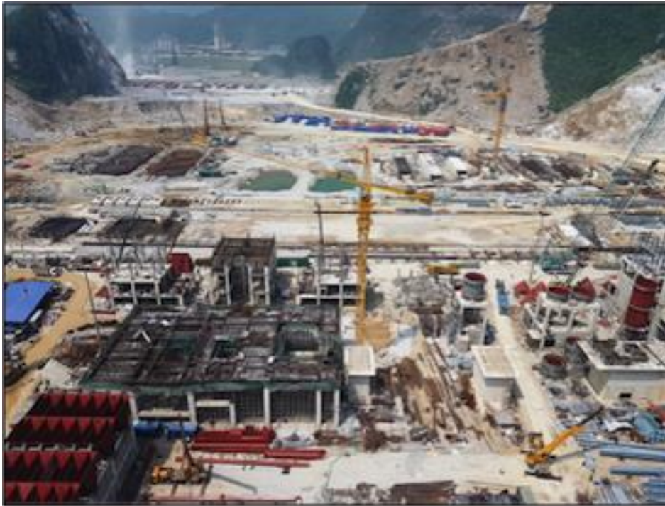
Figure 48: Construction of South East Asia’s largest cement plant Source: Xuan Thanh Group
