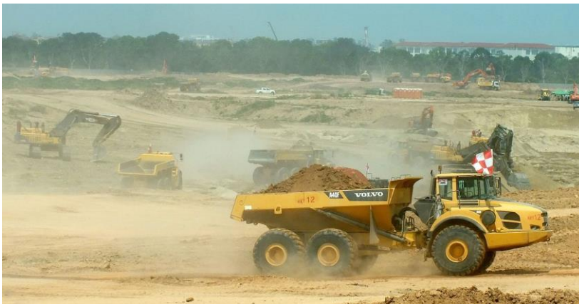
Figure 50: Volvo machines being used by KTC Group Holdings for earthmoving at the site for Changi Airport's Terminal 5
